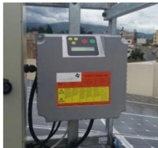
Figura 11. Inversor VASCO solar 212
